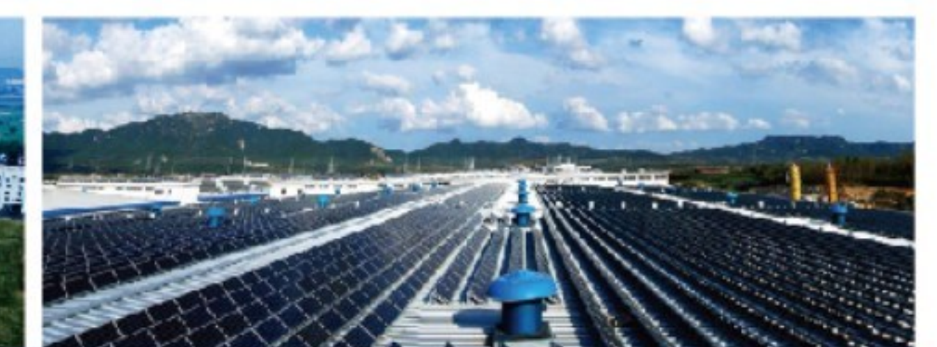
Solar panels arrays
